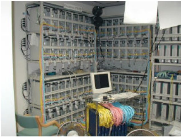
Figure 3: 256-processor high-density Presto II cluster (left)
